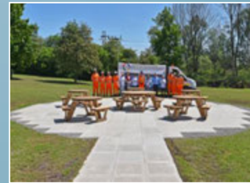
The finished pathway and BBQ area for Friends of Stanley Hall Park, Handforth
